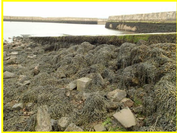
Undercutting of slipway (Asset ref. No. 1221C901C0401C27)
