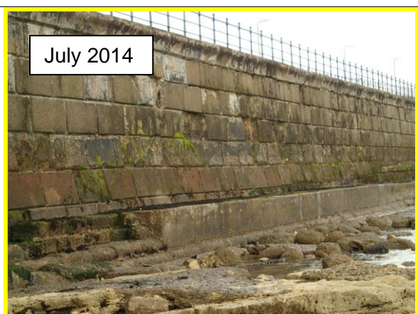
Damage to concrete toe similar to 2012 inspection (Asset ref. No. 1221C901C0303C02)
