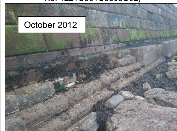
Damage to concrete toe (Asset ref. No. 1221C901C0303C02)
