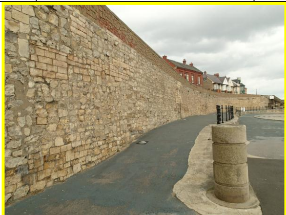
Rear retaining wall at Block Sands with missing mortar in joints and damage to blocks (Asset ref. No. 1221C901C0401C04)
