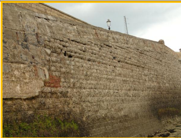
Surface abrasion damage to wall adjacent to ramp showing multiple previous repairs and voids. (Asset ref. No. 1221C901C0303C04)
