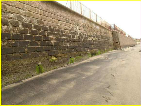
Older concrete block wall in foreground; newer slightly sloping smaller block wall in distance. (Asset ref. No. 1221C901C0401C19)
