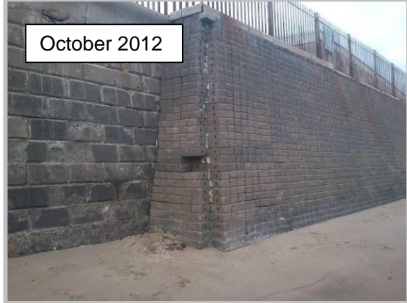
Missing blocks at interface between two sections of wall. Photo from previous report. (Asset ref. No. 1221C901C0401C19)
