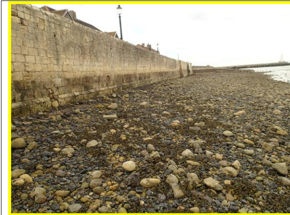
Western section of Town Wall showing low beach levels, (Asset ref. No. 1221C901C0401C35)
