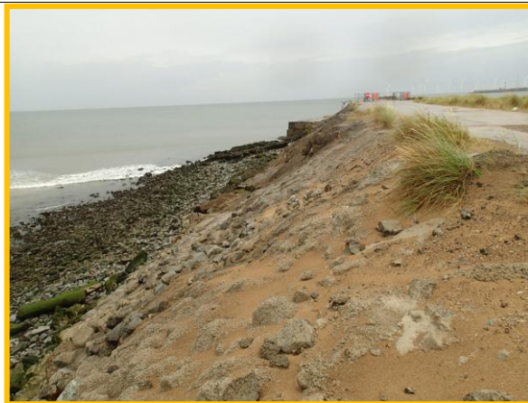
View of patch repairs to north side of breakwater (Asset ref. No. 1221C901C0502C01)
