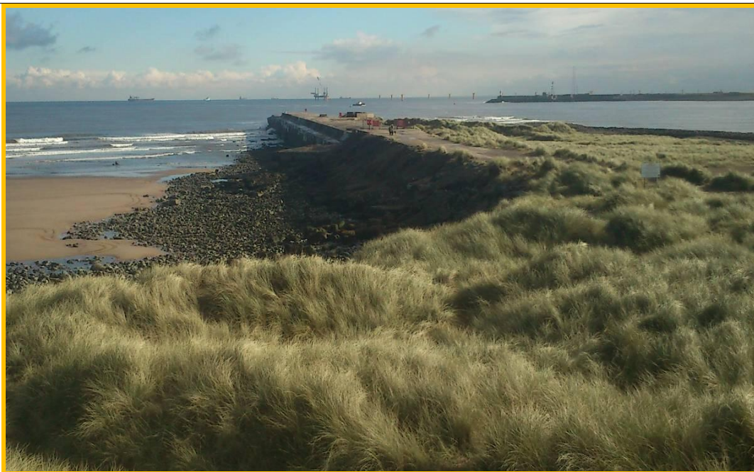
General view of North Gare breakwater, photo from 2012 report. (Asset ref. No. 1221C901C0502C01)
