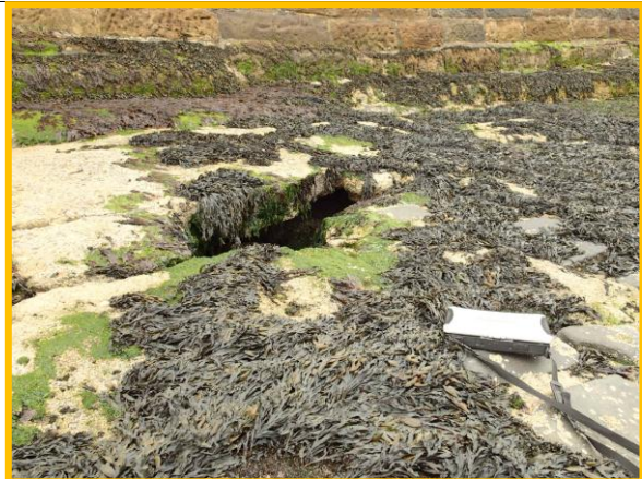
Void in toe apron on north side of North Pier (Asset ref. No. 1221C901C0401C22)
