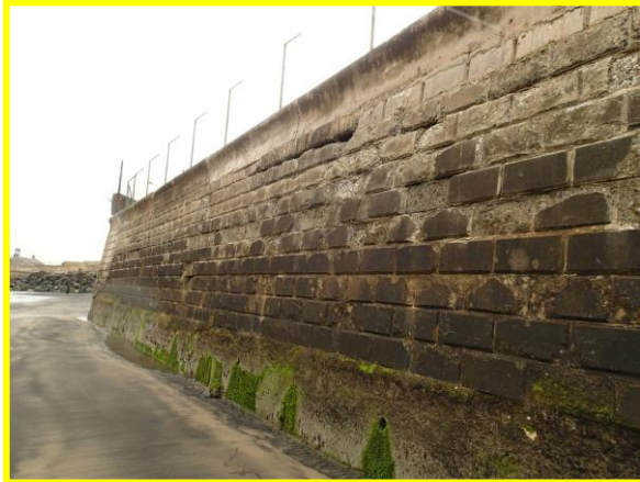
Older concrete block wall has damaged blocks with missing facing. (Asset ref. No. 1221C901C0401C19)
