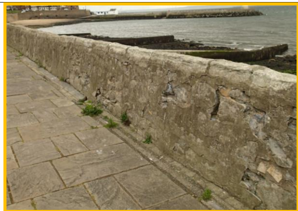
Central part of parapet wall to Town Wall showing missing mortar (Asset ref. No. 1221C901C0401C35)
