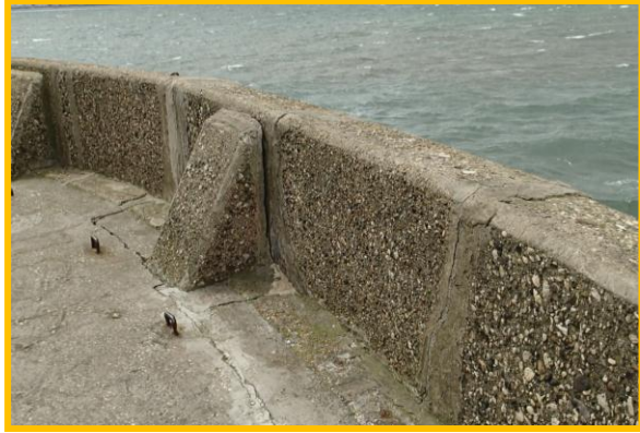
Cracks through deck and crest wall. (Asset ref. No. 1221C901C0401C34)
