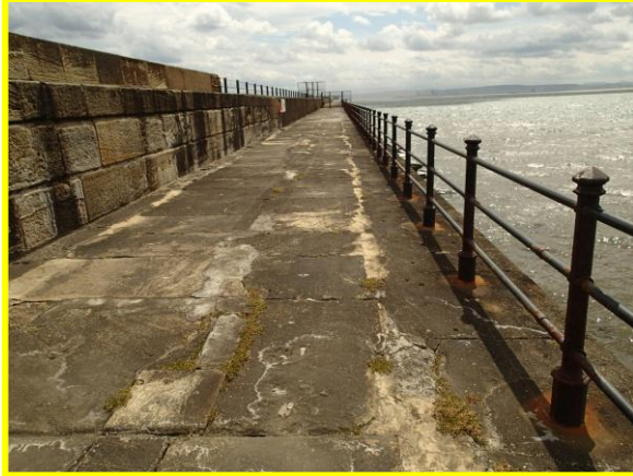
Heugh breakwater promenade, with repairs to gaps between slabs (Asset ref. No. 1221C901C0401C01)
