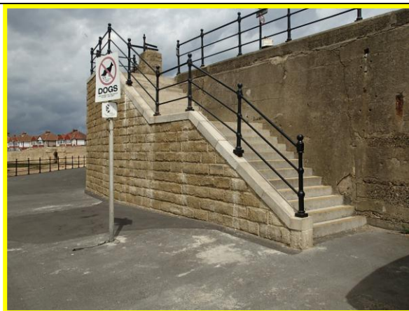
New steps at west end of rear retaining wall, (Asset ref. No. 1221C901C0401C05)
