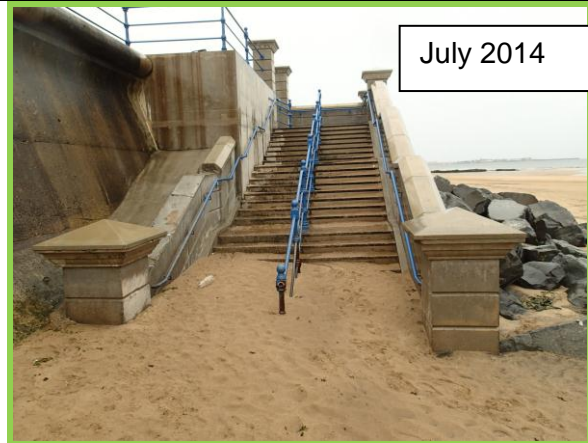
High sand levels at northern steps. Note missing coping stones on wall adjacent to steps (Asset Ref. No. 1221C901C0501C05)
