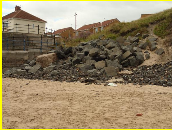
Rock armour at intersection of Marine Drive and slag bank (Asset ref. Nos. 1221C901C0303C01 / 302C03)
