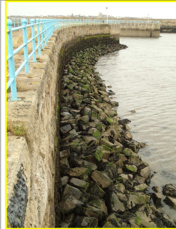
Outer face of Middle Pier, showing rock toe armour. (Asset ref. No. 1221C901C0401C28)
