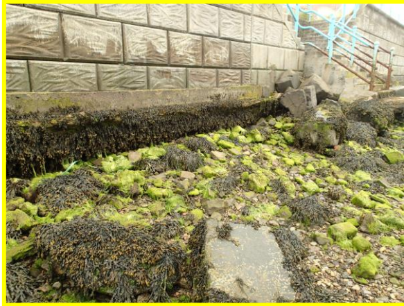
Undermining of toe of wall looking west from slipway (Asset ref. No. 1221C901C0401C27)
