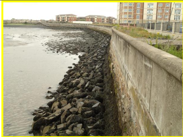
Flood wall and rock toe armour at harbour rear wall (Asset ref. No. 1221C901C0401C29)
