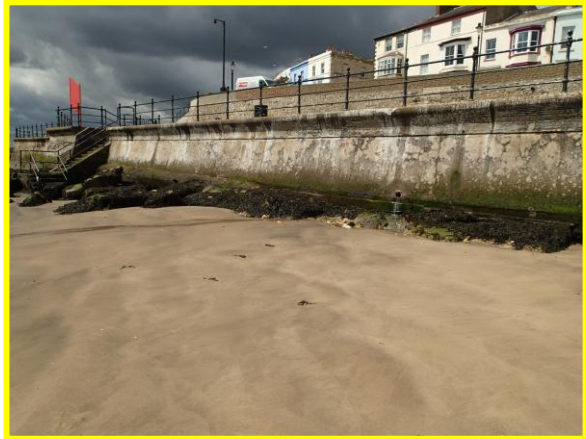
Low beach levels exposing toe at Block Sands wall. (Asset ref. No. 1221C901C0401C04)
