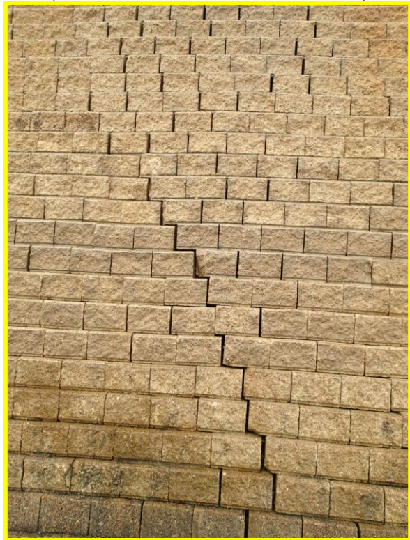
Cracks and opening joints due to movement (Asset ref. No. 1221C901C0401C19)
