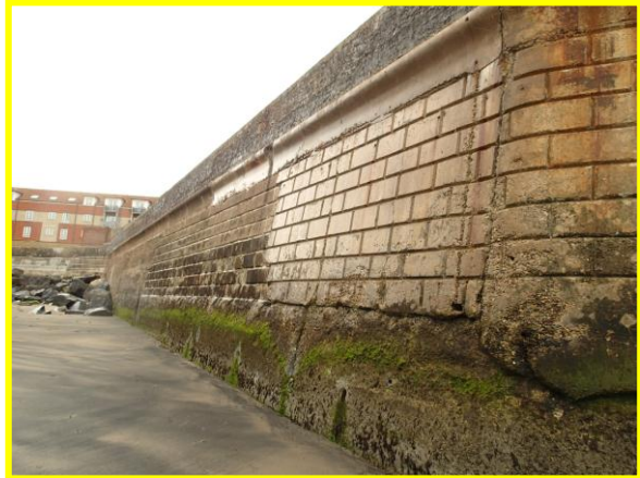
Toe scour and abrasion damage at corner of wall (Asset ref. No. 1221C901C0401C20)
