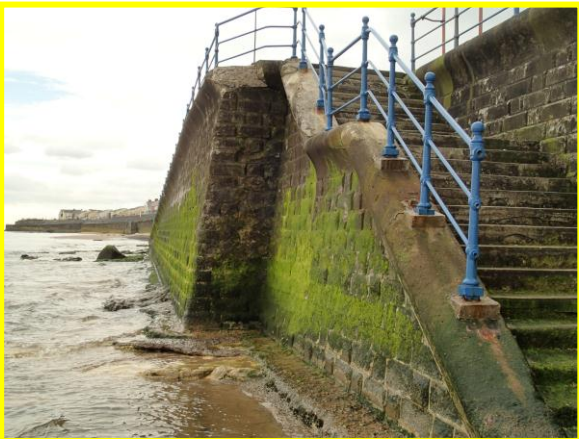
View of blockwork wall with damaged cope and cracking (Asset ref. No. 1221C901C0303C01)
