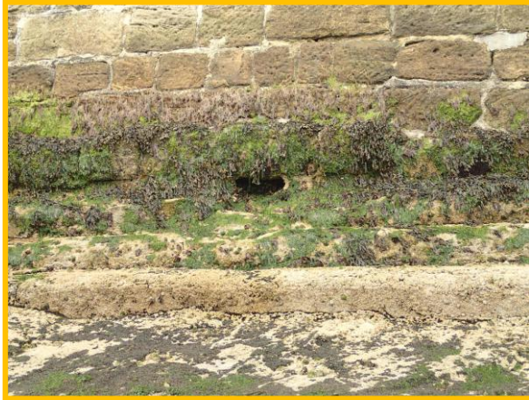
Damaged toe apron exposing void under wall on Middleton Beach side of North Pier (Asset ref. No. 1221C901C0401C22)
