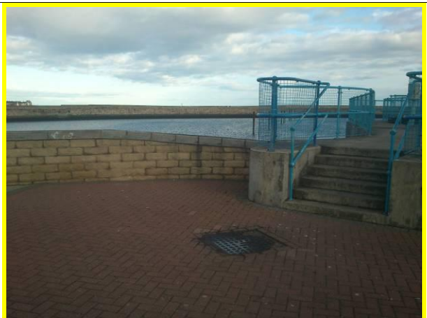
Flood wall tie into lock structure, photo from 2012 report. (Asset ref. No. 1221C901C0401C22)
