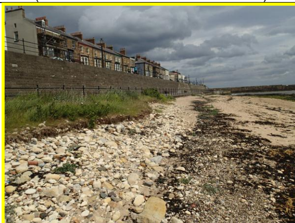
Erosion at edge of cobble beach (Asset ref. No. 1221C901C0401C05)
