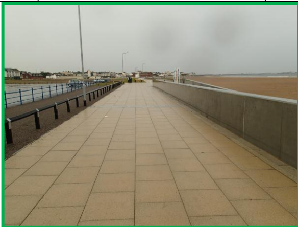
View of new promenade surfacing at car park north of pumping station (Asset Ref. No. 1221C901C0501C03)
