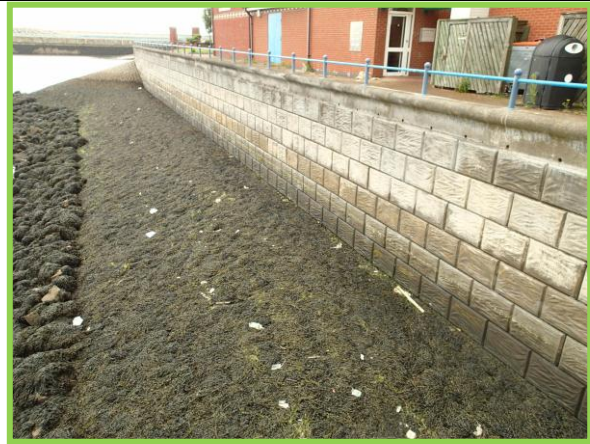
Wall to south side of lock entrance, toe apron covered in seaweed. (Asset ref. No. 1221C901C0401C25)
