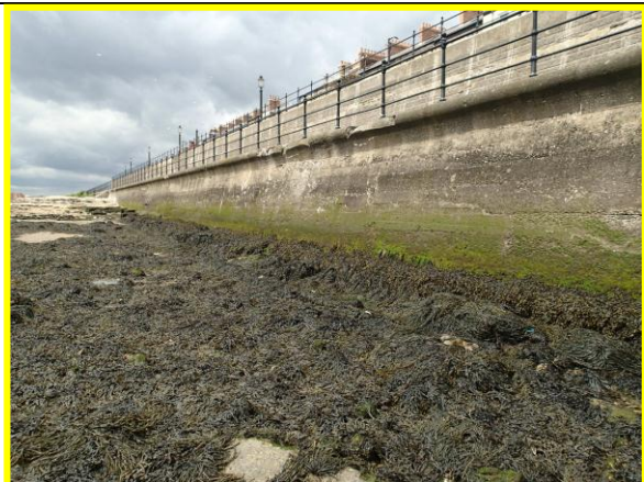
Damaged coping at exposed eastern section (Asset ref. No. 1221C901C0401C05)
