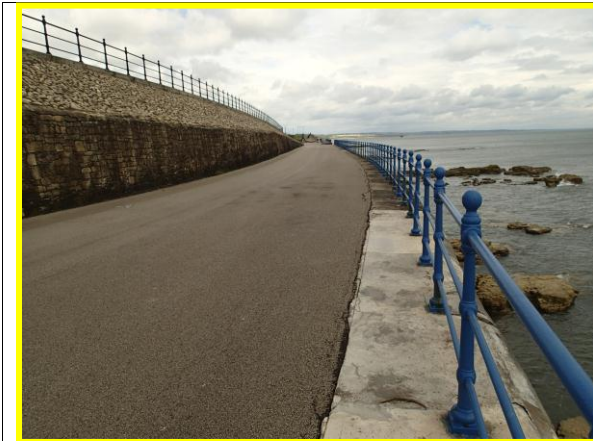
View of promenade and repairs to coping, showing crack adjacent to coping (Asset ref. No. 1221C901C0303C02)
