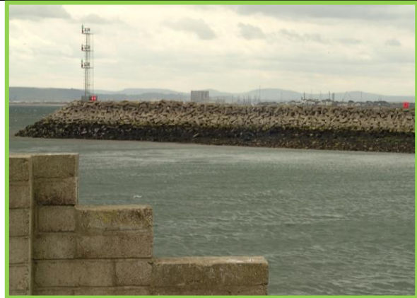
View of Accropode armoured breakwater (Middleton Jetty) from Town Wall. (Asset ref. No. 1221C901C0401C16)
