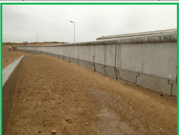
View down ramp access from new seawall at water treatment works. (Asset Ref. No. 1221C901C0501C02)
