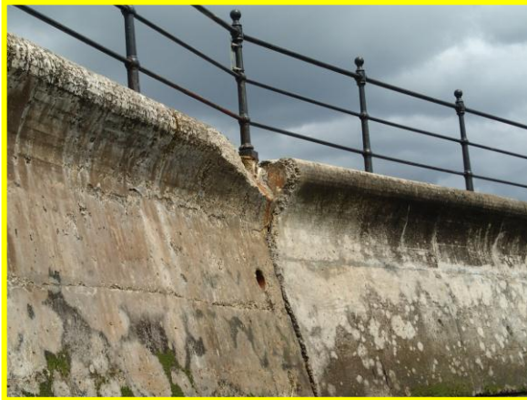
Damage to coping on Block Sands seawall (Asset ref. No. 1221C901C0401C04)
