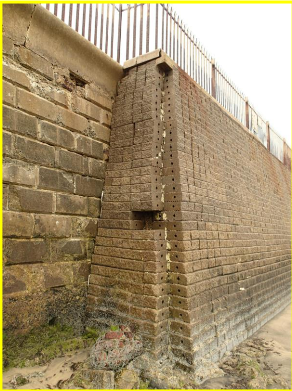
Missing blocks at interface between two sections of wall. (Asset ref. No. 1221C901C0401C19)
