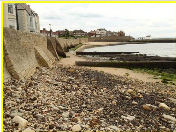
View east along main part of Town Wall. The section in midfield has historically been rebuilt with concrete blocks anchored with steel tie bars which are corroding. (Asset ref. No. 1221C901C0401C35)
