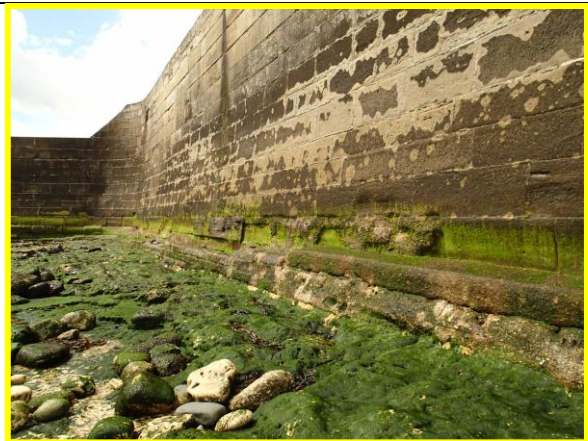
Dressed masonry wall adjacent to Heugh breakwater, showing abrasion to lower wall (Asset ref. No. 1221C901C0401C02)
