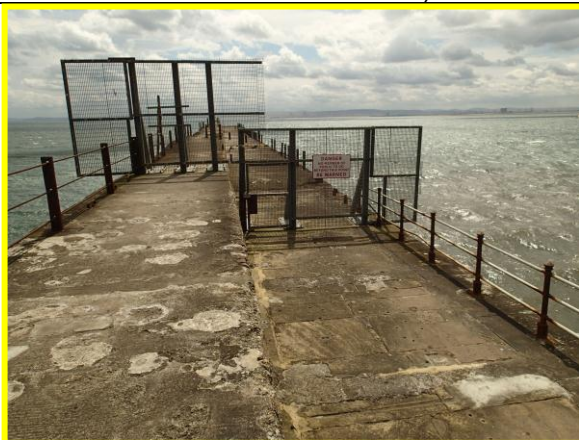
Fencing and warning signs at mid length of breakwater. (Asset ref. No. 1221C901C0401C01)
