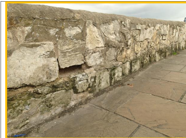
Eastern part of parapet wall to Town Wall showing missing stones and mortar, (Asset ref. No. 1221C901C0401C35)
