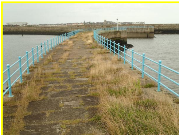
Vegetation growing in between masonry slabs and patch repairs in deck of Middle Pier (Asset ref. No. 1221C901C0401C28)
