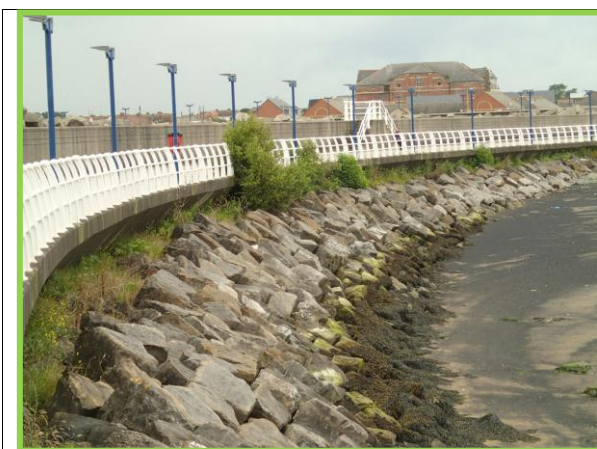
South Pier rock armour on inner face, with vegetation that should be removed. (Asset ref. No. 1221C901C0401C32)
