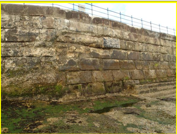
Abraded blockwork wall near Broad Field rd. (Asset ref. No. 1221C901C0303C02)
