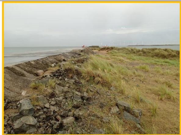
Rubble / slag beach to the south side of North Gare Breakwater. (Asset ref. No. 1221C901C0502C01)
