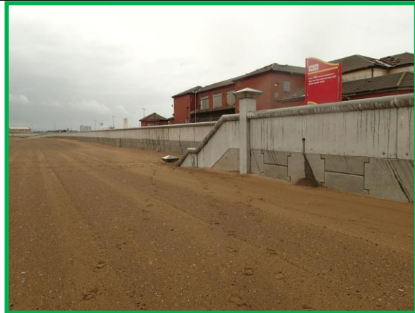
View of new seawall and northern access ramp (Asset ref. No. 1221C901C0401C02)
