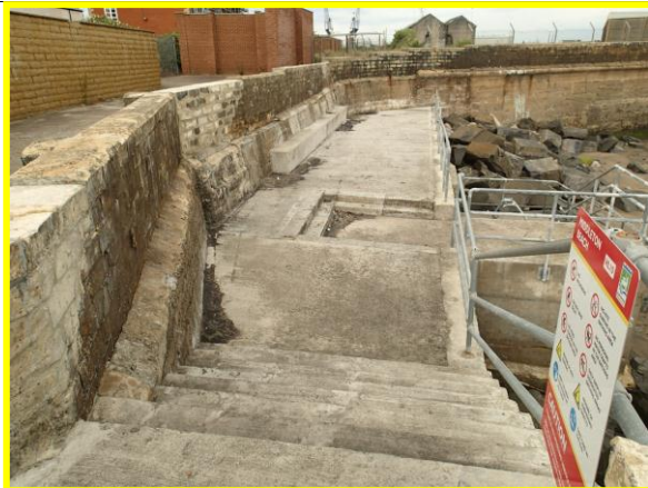
Steps giving access to Middleton beach from root of North Pier (Asset ref. No. 1221C901C0401C22)
