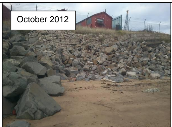
View of Gabion baskets with rock armour. Photo from 2012 report. (Asset ref. No. 1221C901C0401C17)
