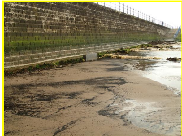
Local repairs to toe have been undertaken but further work is needed to toe and damaged coping. (Asset ref. No. 1221C901C0303C01)
