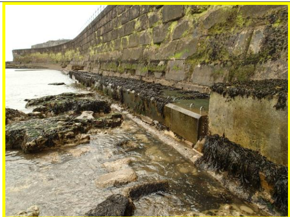
Previous repairs to toe near Sea View Terrace (Asset ref. No. 1221C901C0303C02)
