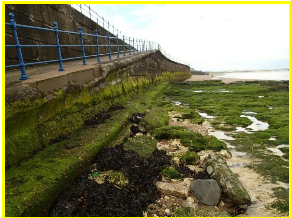
Scour and abrasion at wall toe (Asset ref. No. 1221C901C0303C02)
