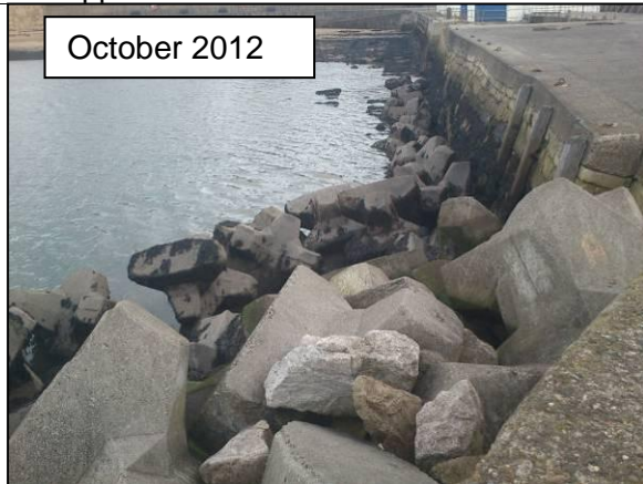
Landward side of Old Pier showing settlement in the (original?) masonry blockwork. (Asset ref. No. 1221C901C0401C06)
