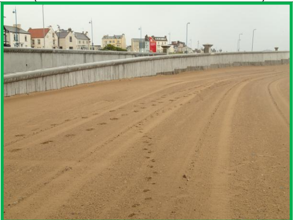
Recently constructed new beach access ramp and seawall at south end of main seawall. (Asset Ref. No. 1221C901C0501C05)
