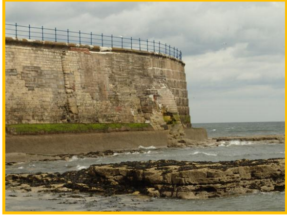
Damage and missing blocks at south of headland (Asset ref. Nos. 1221C901C0303C04 & 1221C901C0303C04)
