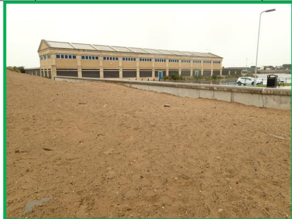
Tie in of seawall at water treatment works. (Asset Ref. No. 1221C901C0501C02)
