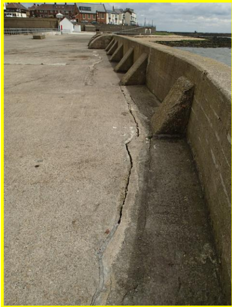
Cracking alongside crest wall (Asset ref. No. 1221C901C0401C34)
