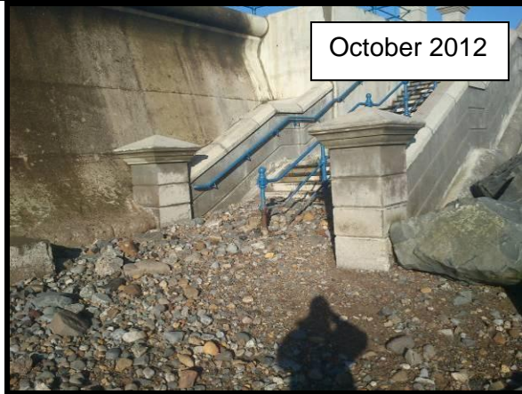
High cobble beach level adjacent to rebuilt northern steps in 2012. (Asset Ref. No. 1221C901C0501C05)
