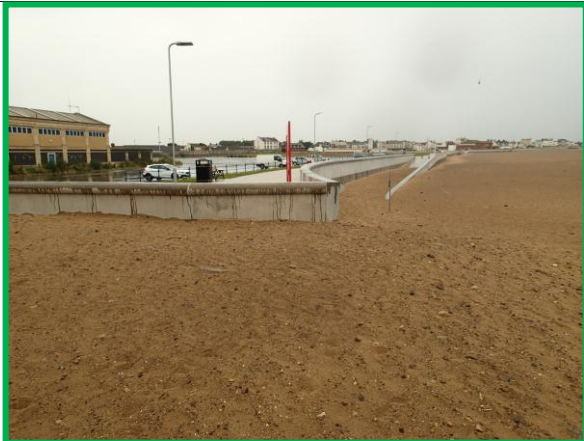
Southern end of new seawall at water treatment works. (Asset Ref. No. 1221C901C0501C02)
