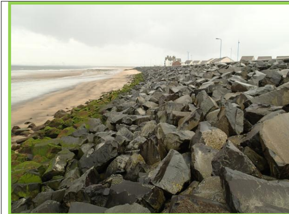
Rock armour in good condition near north end of Seaton Carew (Asset ref. No. 1221C901C0401C33)
