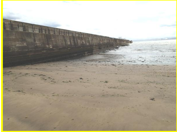
South side of landward end of Heugh breakwater (Asset ref. No. 1221C901C0401C01)
